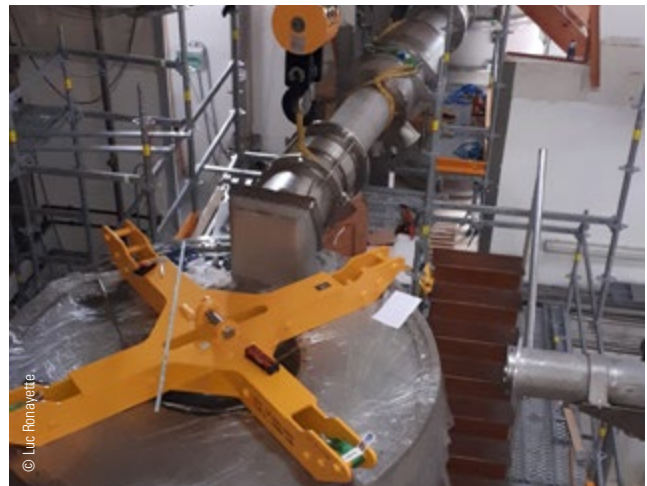
› Figure 3: Trial assembly of the cryogenic line (contractor Cryo Diffusion) connecting the cryogenic satellite in the back to the superconducting magnet cryostat in the front.
