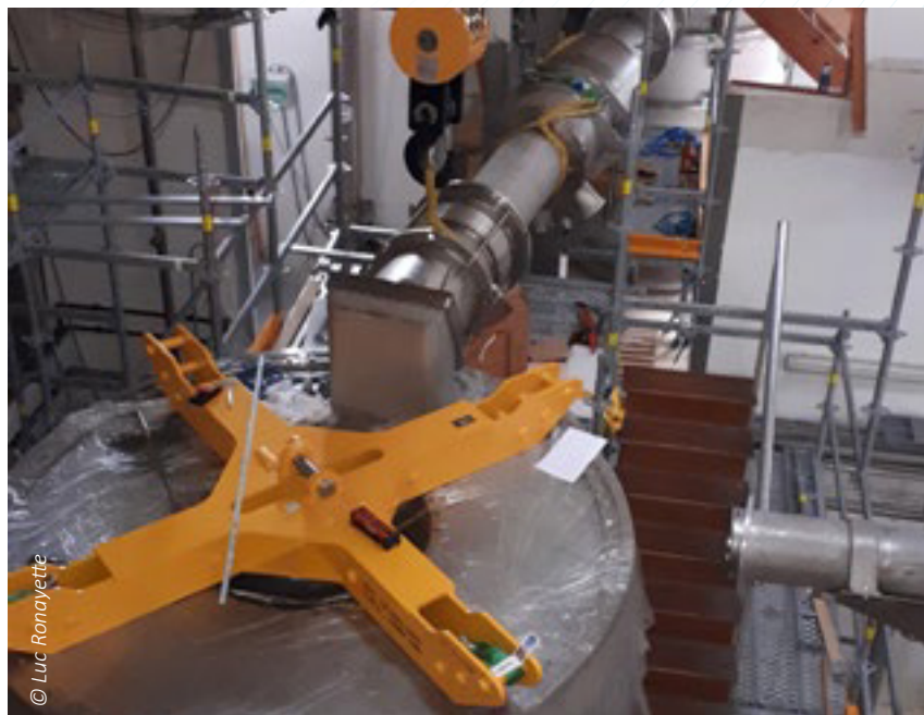
Trial assembly of the cryogenic line (contractor Cryo Diffusion) connecting the cryogenic satellite in the back to the superconducting magnet cryostat in the front.
